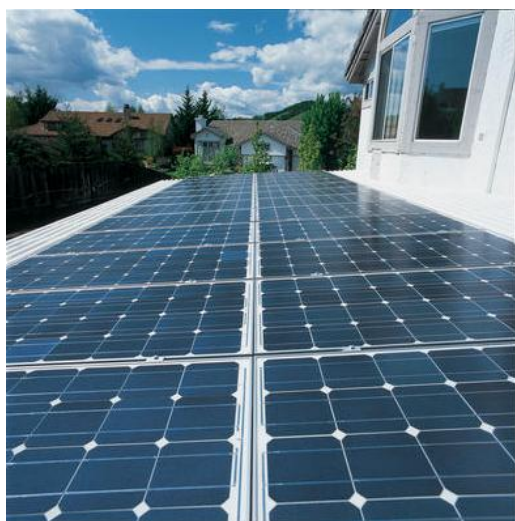
Solar photovoltaic cell panels integrated into a back porch awning
