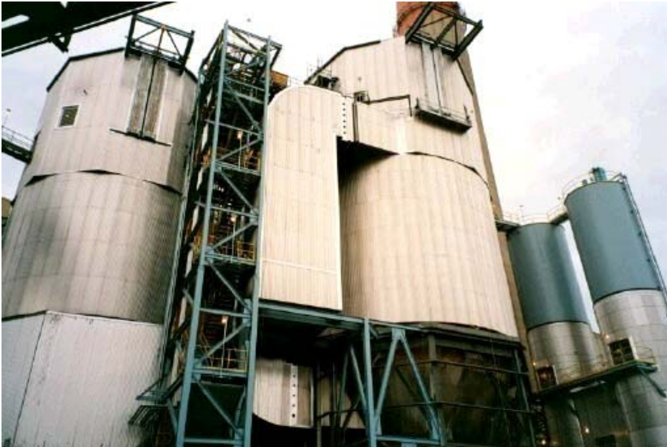
SO 2 scrubber for a 150MW unit at Cherokee Station in Denver
